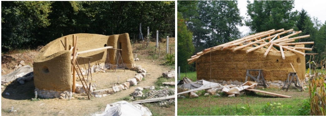
Figure 10. (Half)greenhouse, Banja Luka, Republic of Srpska, Bosnia and Herzegovina (arch. papers first author, 2011-2014) during construction of the heat-retaining northern wall and roof structure. Materials: earth, straw, wood, glass. Photo: paper's first author
