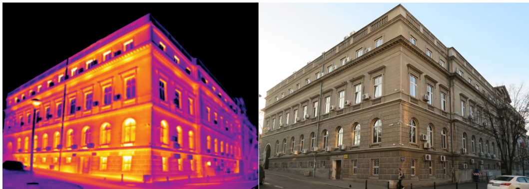
Figure 3. Thermal imaging and photograph of the street facade of the building of the City Municipality of Zemun. Heat losses are evident in the area where concrete beams are - over windows and in the area of window openings
