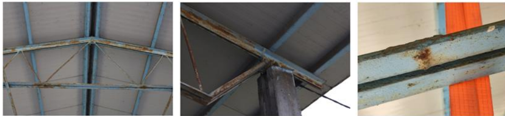
Figure 2. Typical examples of corrosion on steel members and welded joints (photography by author).
