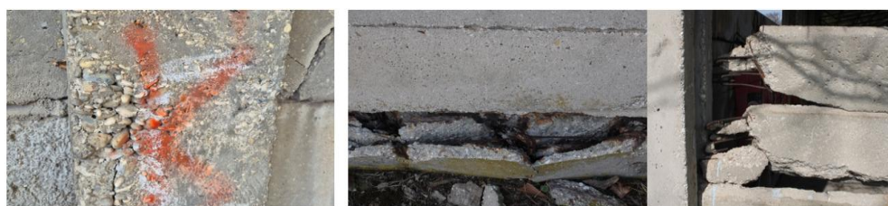
Figure 4. Segregation of concrete in the columns (left) and deterioration of non-structural elements (parapet walls) (right) (photography by author).
