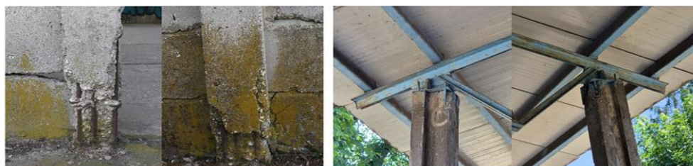
Figure 3. Spalling of concrete cover in column lower zones (left) and upper zones near the anchor plate (right) (photography by author).
