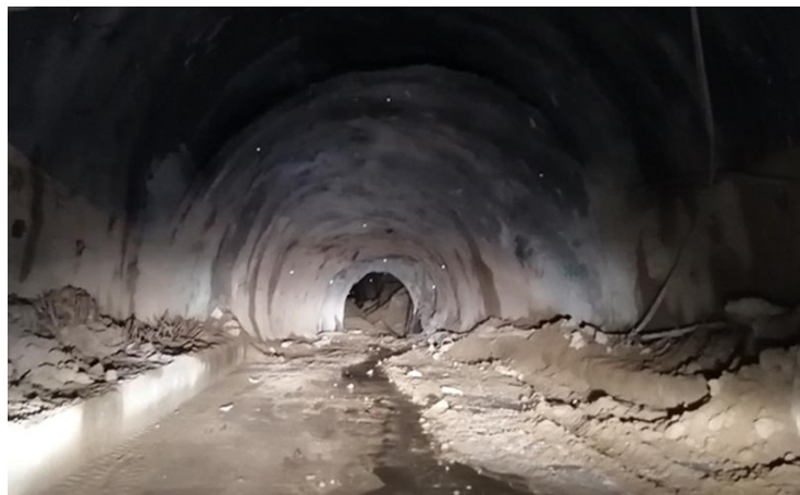
Figure 2. Reduced profile, through the collapsed material of the Ibarac tunnel (photography by author).
