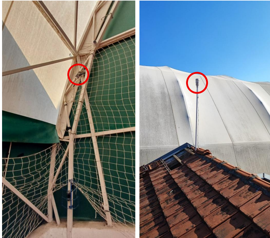
Figure 6. Internal and external part of the meteorological station (source: photographs by authors).
