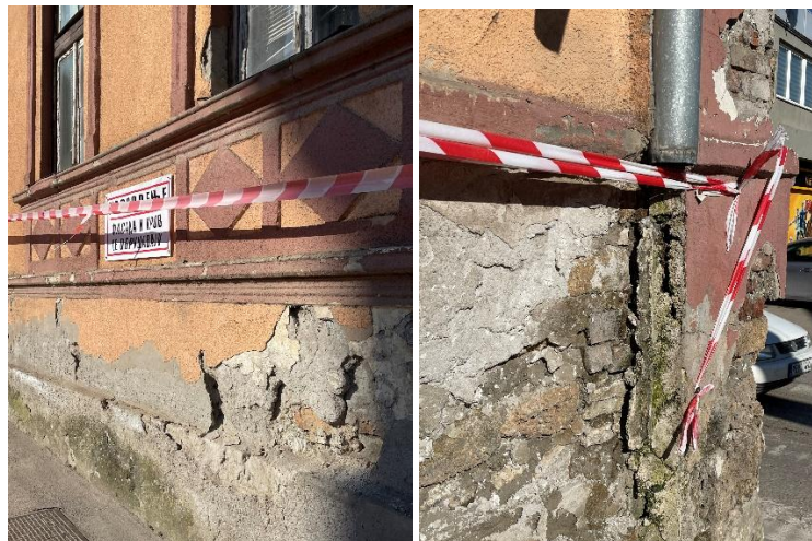
Figure 2. Current state of foundations (photography by author)
