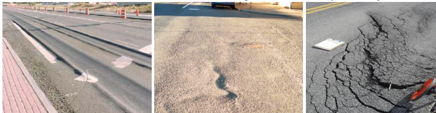
Figure 6. Distresses of pavement at the intersection area (left: rutting, middle: shoving, right: slippage cracking)
