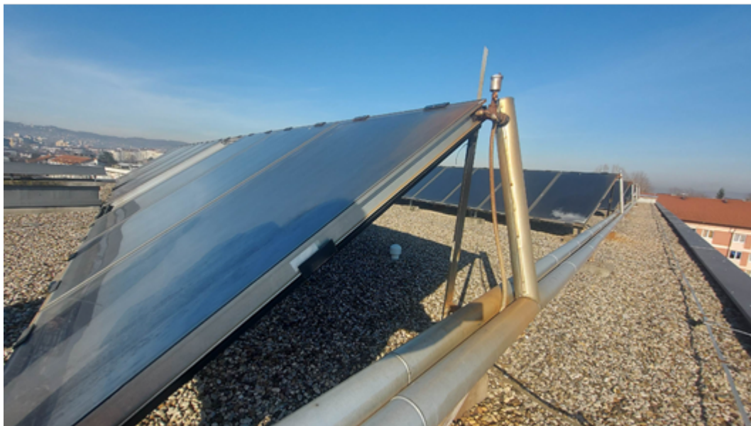
Figure 2. Solar thermal collectors (STC) on the roof of Student Dormitory
