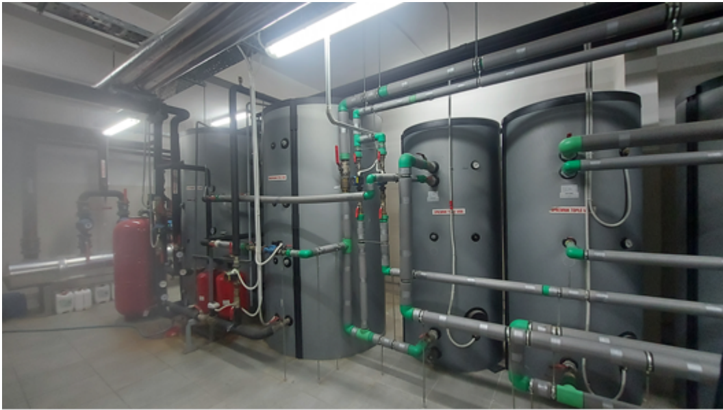
Figure 3. Boiler rooms at the Student Dormitory
