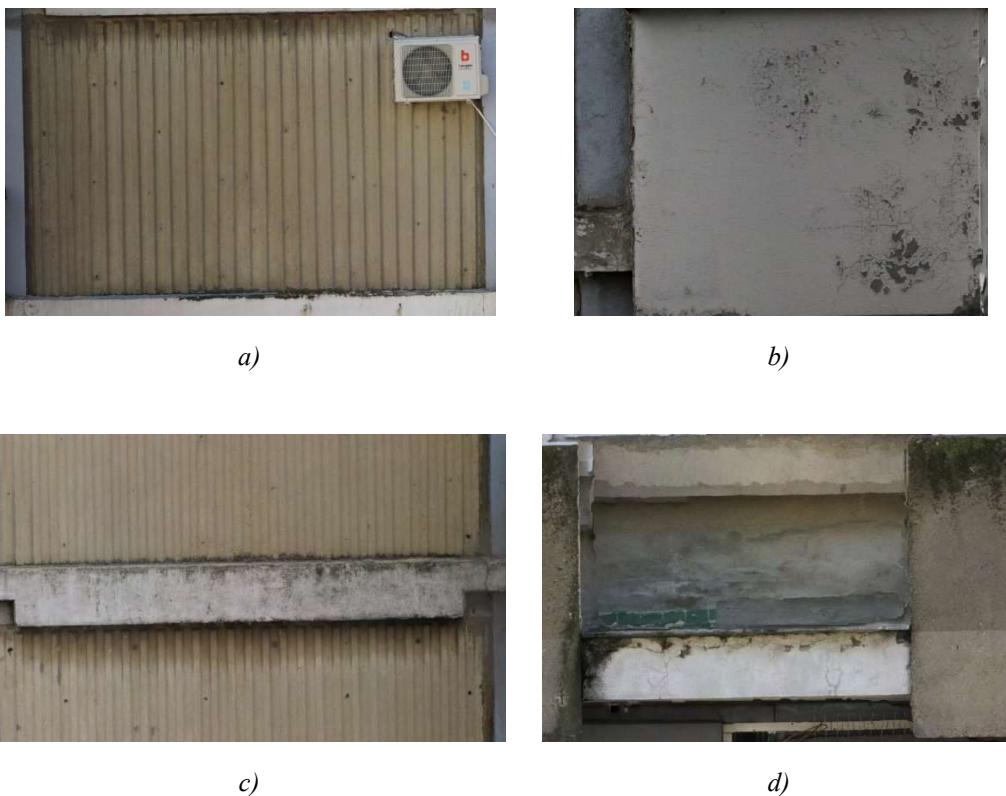
Figure 5. Cracks on the facade
