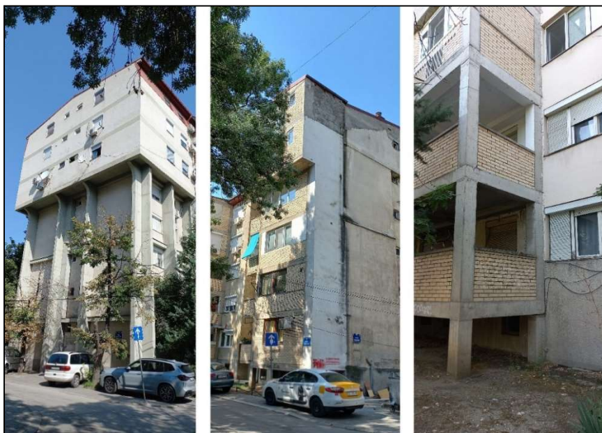
Figure 6. Buildings with mixed structure with use of expansion joints. Source: photos by K. Edip.
